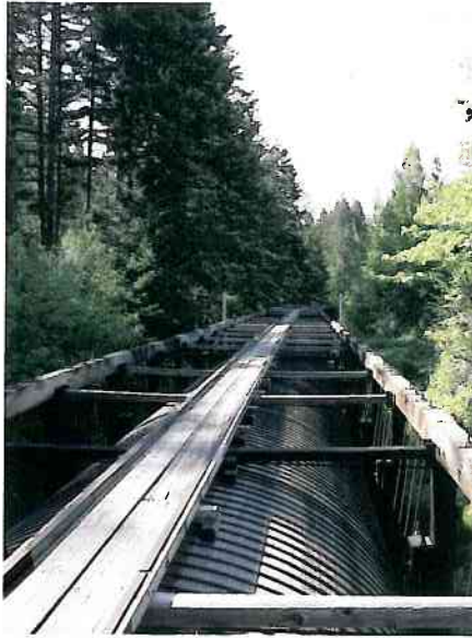
This enclosed flume connects the dam with the powerhouse
